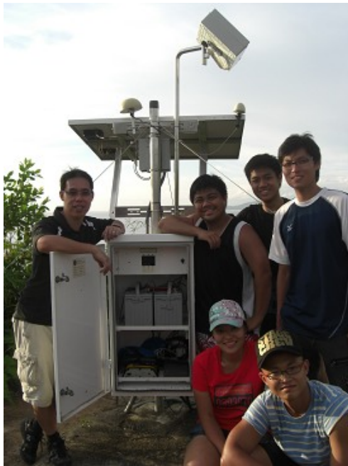
Fig. 6. Installation of upgraded sensors and instrumentation at PSKI, weather stations, tilt meters, accelerometers (for seismic measurements), gas sensors, tide gauges (for sites close to the shore) and digital cameras. The site cabinet architecture, communications system arrangement, power budget and ACeS bandwidth preclude any of these. In fact, much legacy SuGAR network hardware has been superseded by lower power, more reliably and capable alternatives, the common eventual fate of many pioneering systems.
